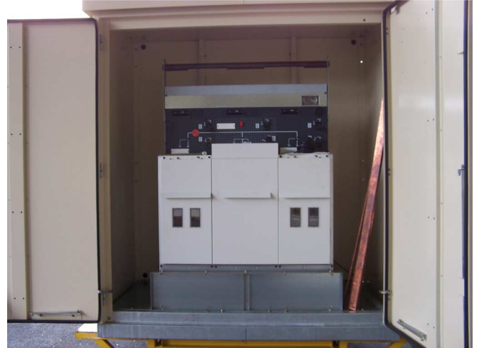
Fig. 1. MV cubicle photo from a test setup.
