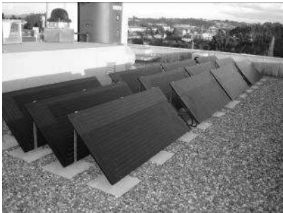
Figure 3. Hot water solar collectors (thermodynamic system).
