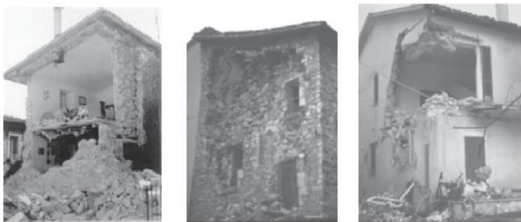
Figure 5 Out-of-plane mechanism observed in unretrofitted buildings [7]
