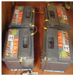
Figure 7. Used lead-acid batteries (48 V – 44 Ah).
