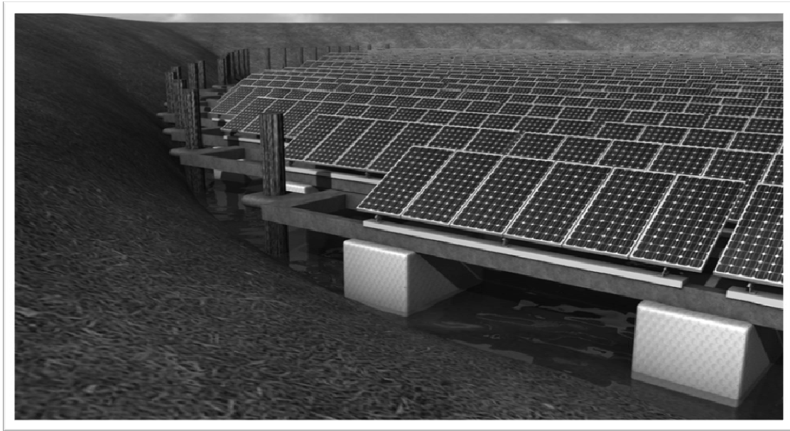
Figure 18. Thick film crystalline panels floating on retention ponds at the Turkey Lake Service Plaza
