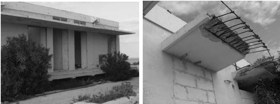
Figure 2. Existing deteriorated structure & reinforced concrete elements on façade prior to repair.
