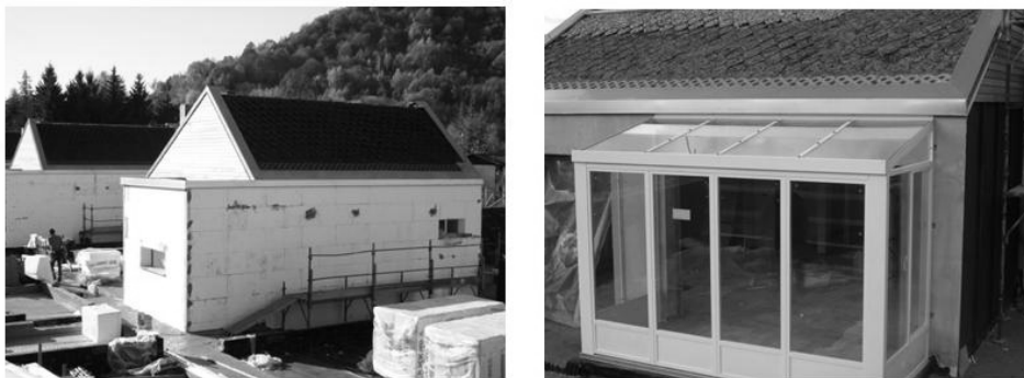
Figure 5. Two pictures during the construction phase: from left to right, the north and the south façade with the conservatory space.
