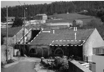
a. 1 st Collapse (2000)
