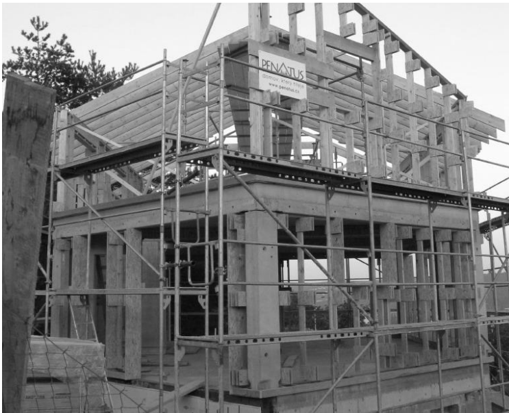
Figure 7 Timber frame structure on the top of RC precast part. Fixing of timber external wall.
