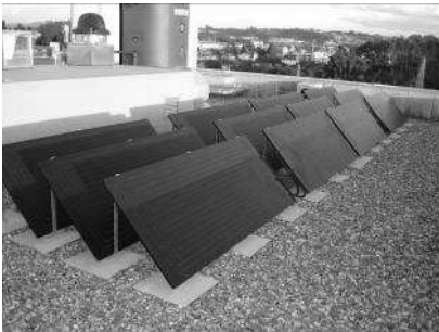
Figure 3. Hot water solar collectors (thermodynamic system).
