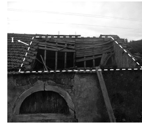
c. 3 rd Collapse (2009)
