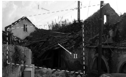
b. 2 nd Collapse (2007)
