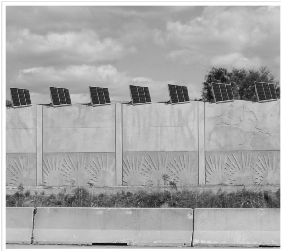
Figure 16. Top mounted thick film crystalline panels located on top of the noise walls along the Florida Turnpike in the vicinity of the Turkey Lake Service Plaza
