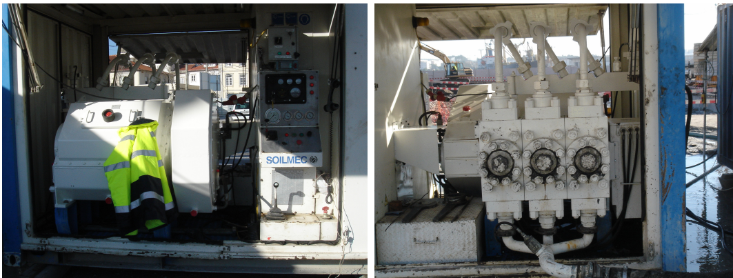
Figure 3.10: Pump station (equipment used in Multiusos - Viana do Castelo)
