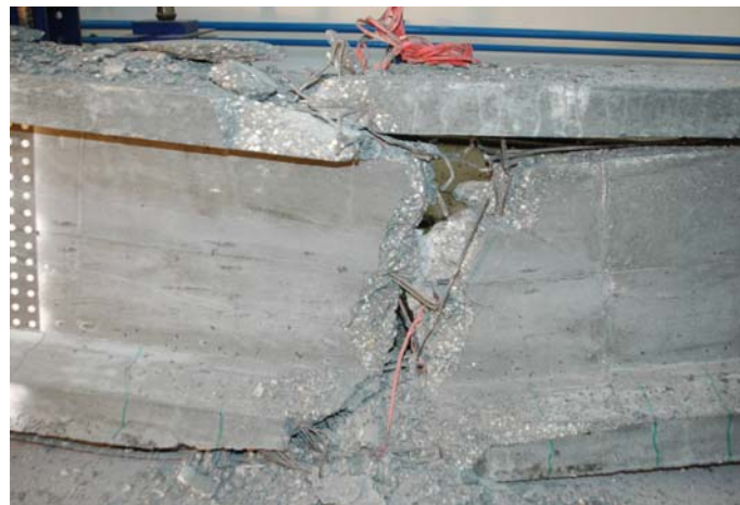
Figure 9: Failure mode observed in girder STR_PRE.
