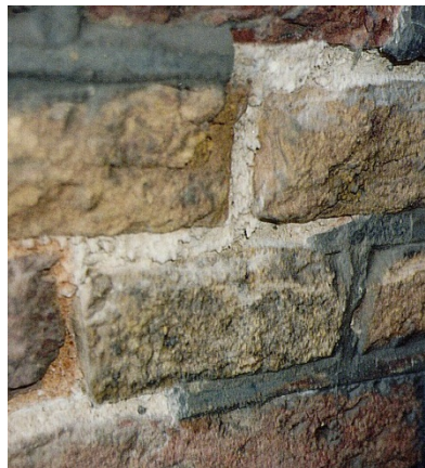
Fig. 6 Push-out of cement re-pointing due to crystallization of salts at the interface of new pointing and old bedding mortar.
