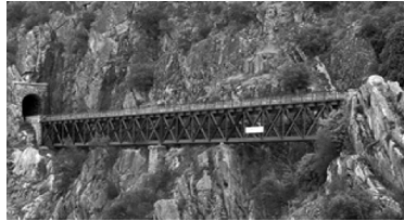
Figure 6 – Tunnel and Viaduct of Presas in Tua line at the km 1 (Meireles, 2011)
