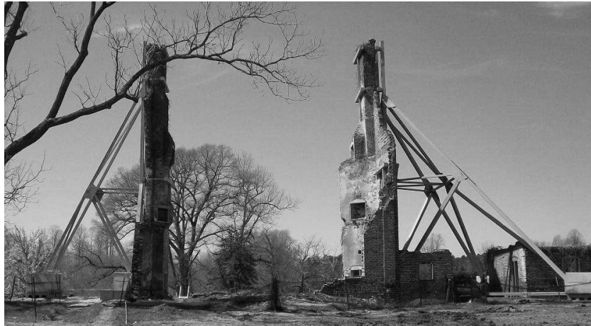
Figure 1: Additional bracing structures visibly damaging the authenticity of ruins in seismic area
