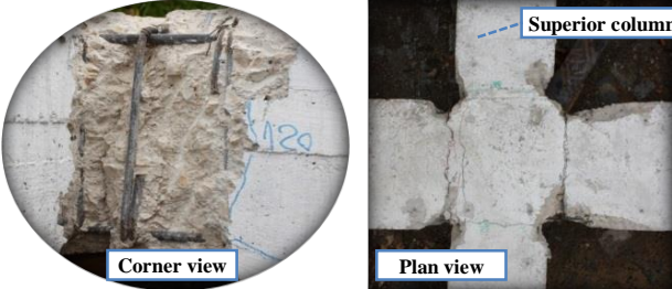
Figure 10 : Level of damage in the prototype before its repairing
