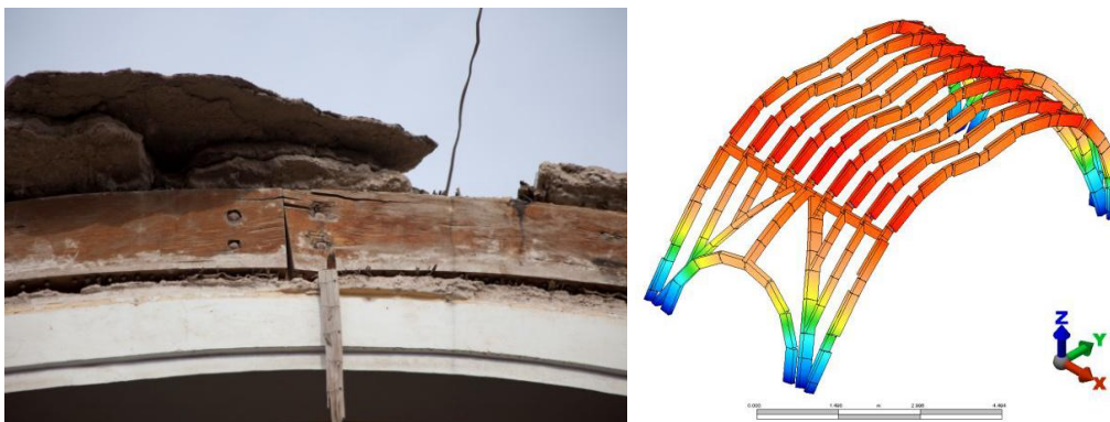
Figure 7: a) In situ plain lap joint for planked arches; b) F.e. model of a timber vaults
