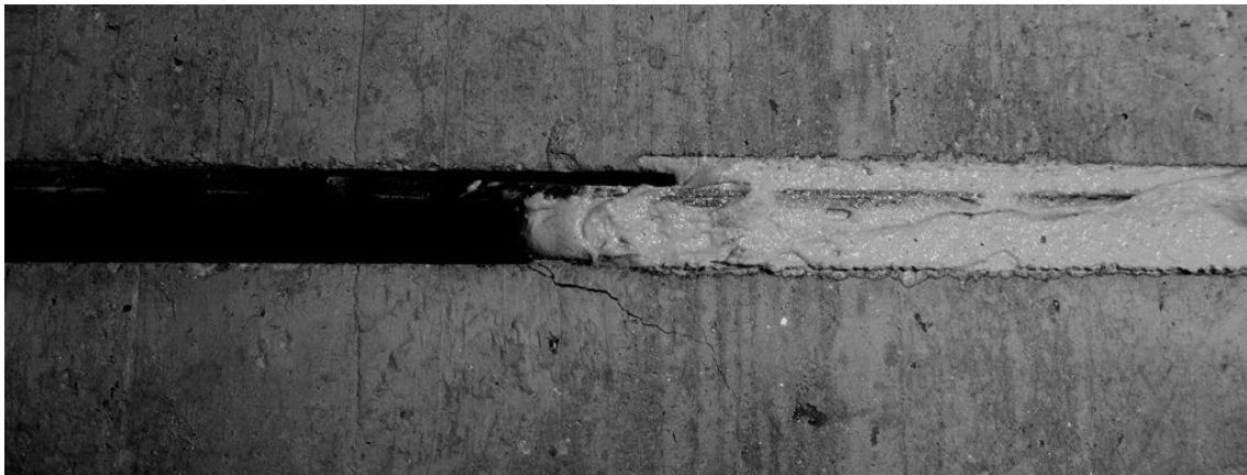
Figure 124 – Crack in the free-end of the active end side – S3_40%.
