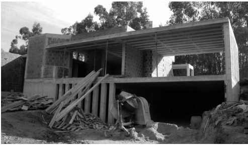
Fig. 4 - Contemporary house with steel reinforced concrete structure, hollow brick walls and beam and pot slabs.
