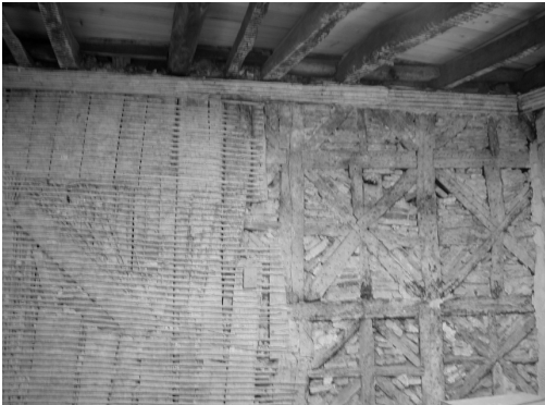
Fig. 5 - “Taipa de fasquio” / “Taipa de rodizio” – Wattle and daub / Daub and half-timbered techniques in a same wall, on a traditional house located in Guimarães historical center, Portugal.
