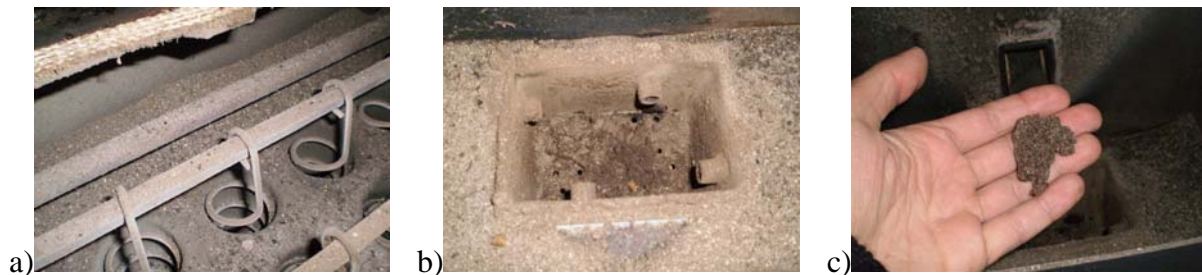
Figure 3. Ash problems in the boiler by the FRWP: a) fouling in the heat exchanger; b) slagging and obstruction of the air inlets of the grate; and c) slagging of the ash fusion.
