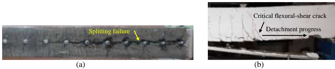
Figure 8- Propagated damages at the end of the test of (a) FB2_B (bottom view), and (b) FB2_G
