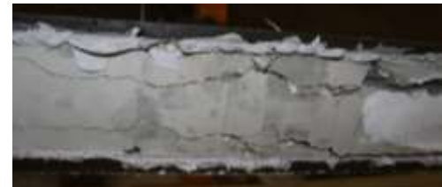
j) Crack pattern in the bottom surface at failure load of SP-3L45 beam
