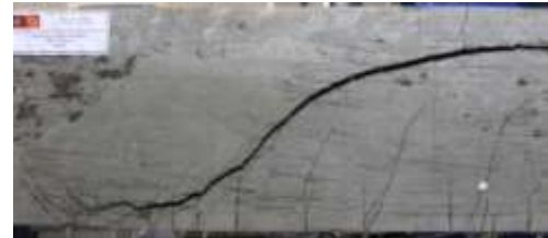
f) Crack pattern at failure load of the SP beam
