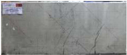
i) Crack pattern in the lateral surface of SP-3L45 beam at the load level of 123 kN
