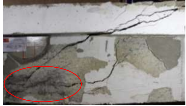
b) Final crack pattern of the SP-3L45 beam when HCP was peeled off after the test
