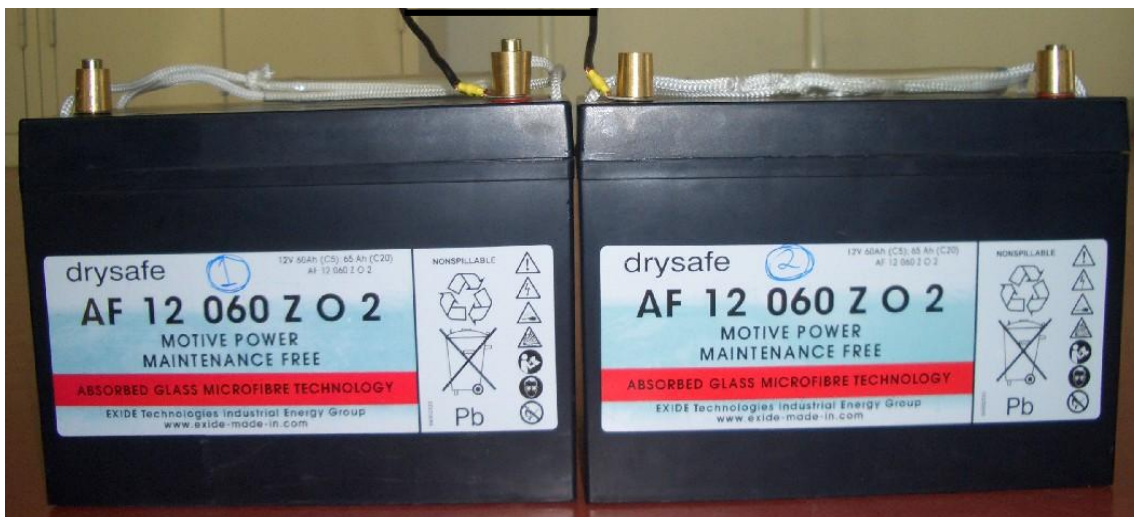
Figure 23 – Serial Connection between two Exide batteries
