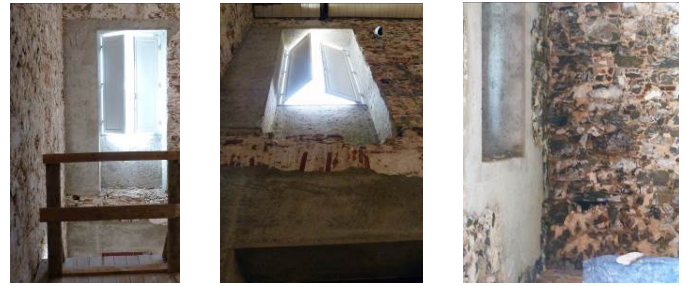
Figure 14. Different parts of the back wall partially reconstructed close to the connection with the longitudinal walls.
