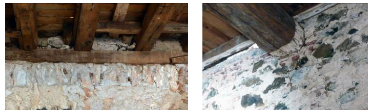
Figure 10. (left) Timber floor beams resting on transverse timber plate (right) Timber floor beams piercing the walls.
