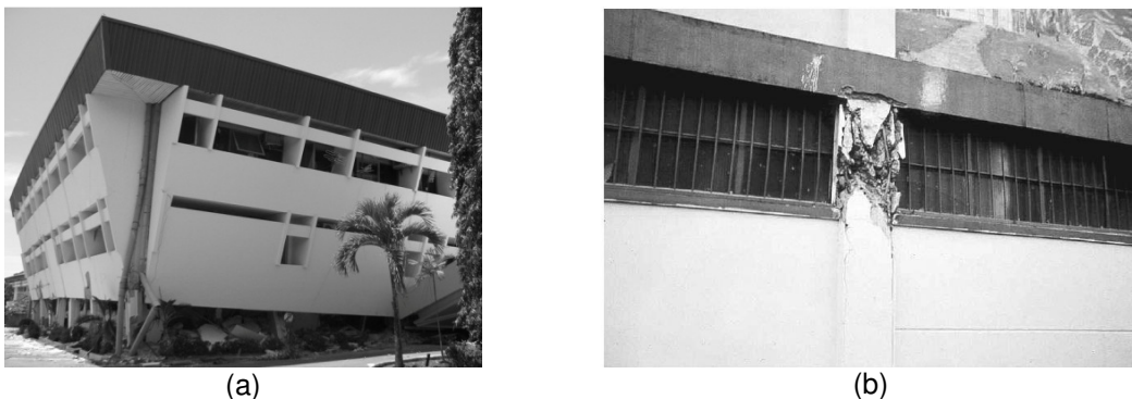
Figure 1: Negative effects of infill panel in structure; (a) soft story mechanism [5], (b) short column mechanism [6].
