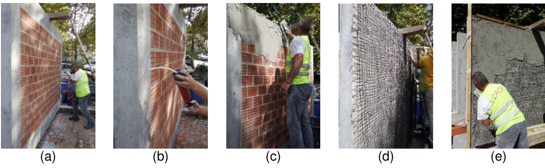
Figure 5: TRM retrofitting technique; (a) drilling the holes (b) cleaning the holes (c) casting thin-layer rendering (d) installing meshes on rendered surface by using shear connectors (e) final rendering and rectifying the rendered surface.
