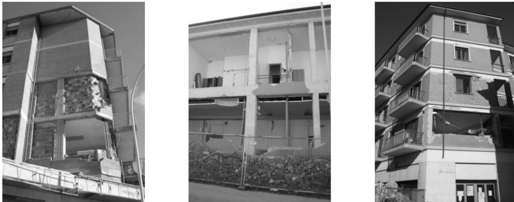
Figure 1: Partial and complete out-of-plane collapses of infill walls during the L'Aquila earthquake (2009), Italy, which is a recurring phenomenon.
