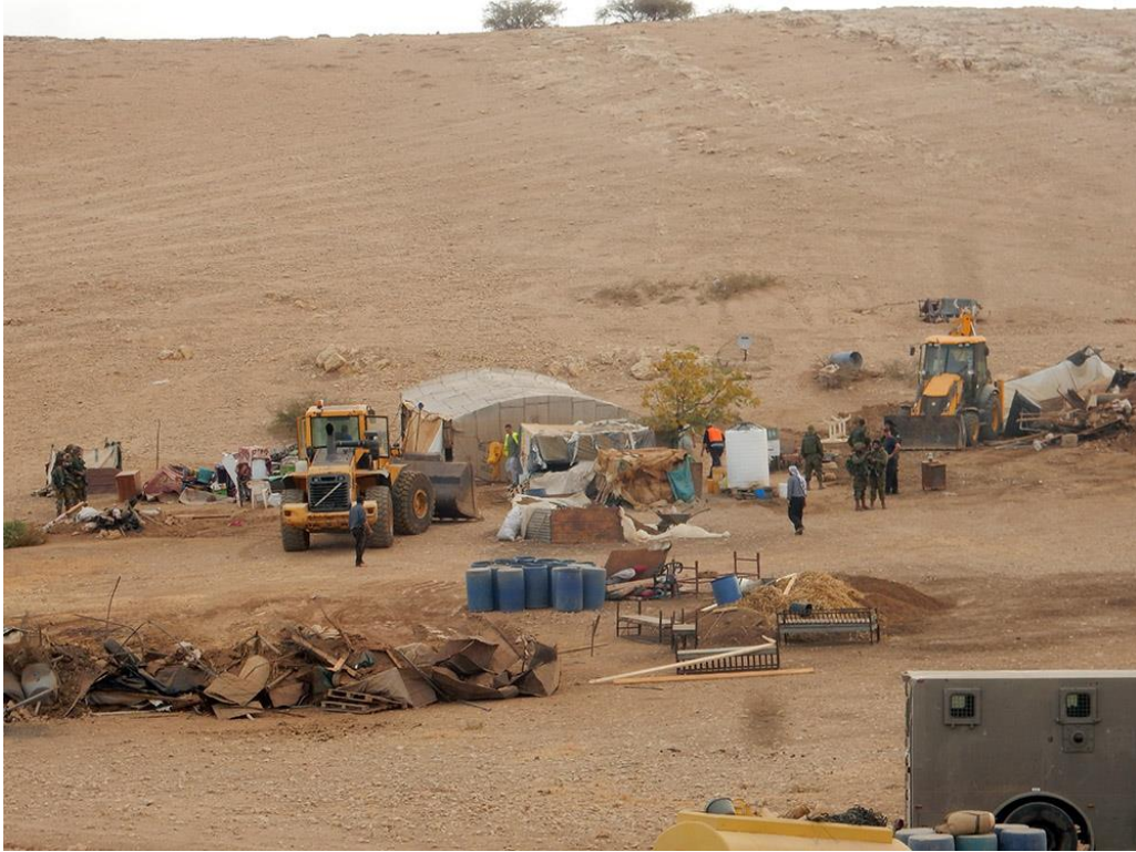
Fig. 5-13: An Israeli bulldozer demolishing a Palestinian building in the Jordan Valley (B'Tselem, 2016)
