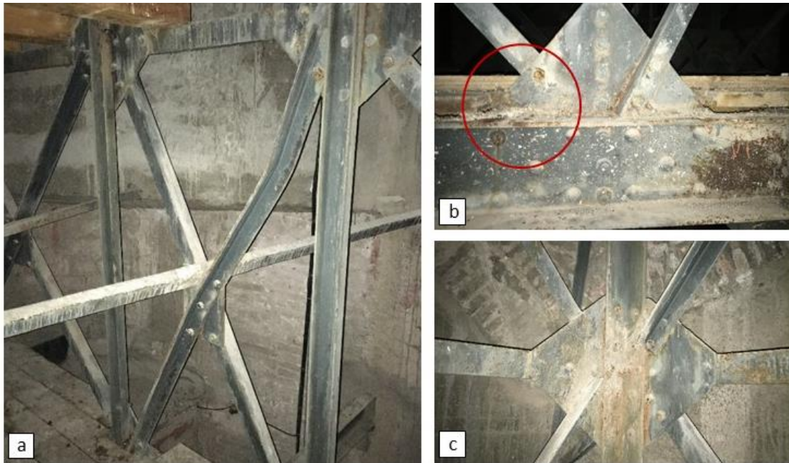
Figure 4-10 Metal structure decay: a) deformations, b) corrosion of connectors, c) corrosion of profiles
