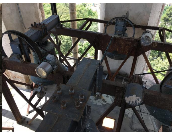
Figure 4-7 Upper part of the metal structure, in correspondence of the belfry, where bells are located
