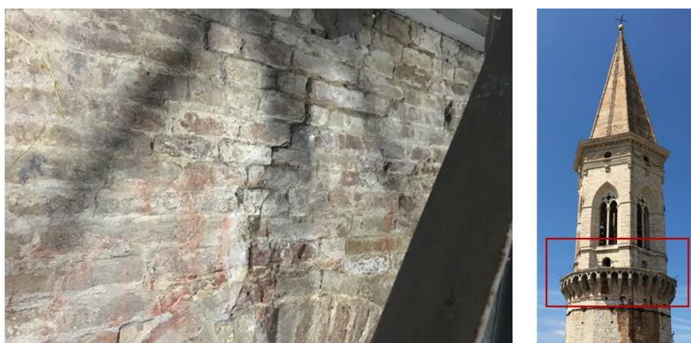
Figure 4-1 Crack in the lower part of the belfry
