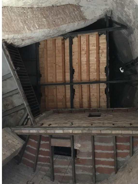
Figure 3-14 Interior of the shaft: partially demolished masonry stairs, lower part of the metal structure, room of the clock's mechanism
