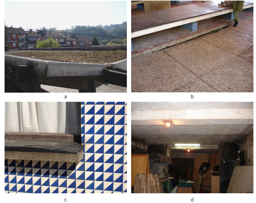
Fig. 47 2015 Survey of the Municipal Market of Santa Maria da Feira; damages affecting various elements.
