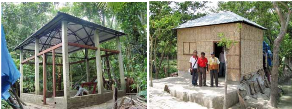
Fig. 21: Core shelter following Cyclone Sidr in Bangladesh, 2007. The core shelters were built by contractors and selection of families was through a lengthy transparent process. Left shows the frame of the structure. Source: Xavier Génot, IFRC.
