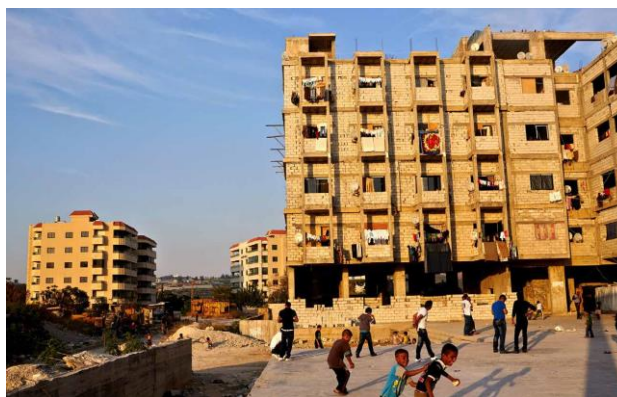
Fig. 12: Unfinished building inhabited by Syrian refugees, Duhok city, Kurdistan Region of Iraq. This type of skeleton poses a real challenge in terms of ensuring safety and security. Photo by: Wan Sophonpanich. Source: (IFRC, UN-HABITAT, and UNHCR 2014, 30).
