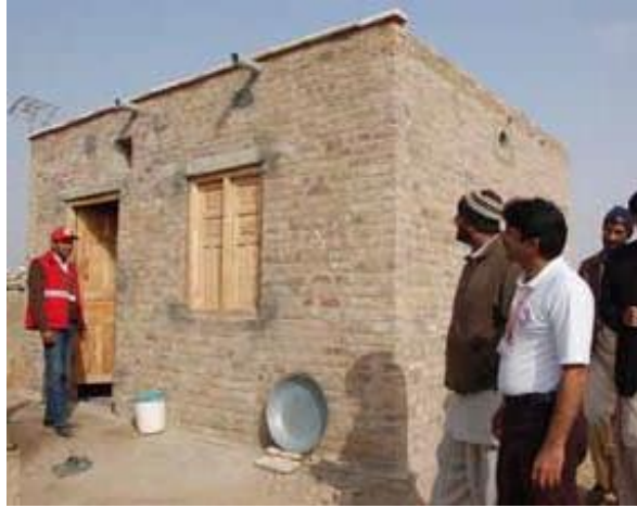
Fig. 20: One room shelter following a flood in Pakistan, 2010. Source: (Ashmore and Treherne 2013, 2:87).
