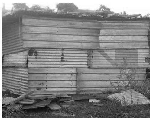
Fig. 15: Poor quality shelter characteristics in Fiji following Tropical Cyclone Evan 2012. Source: Habitat for Humanity Fiji.
