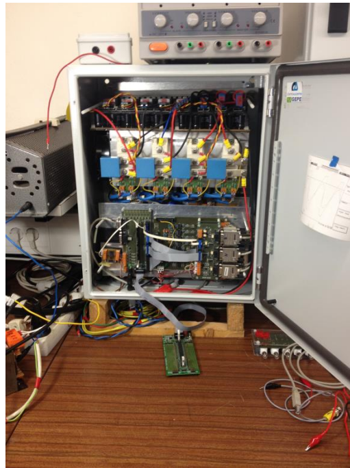
Figure 6.1 - Integrated converter to which the project was migrated.
