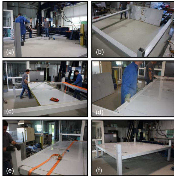
Fig. 10. Stages of the assembling process:(a) placing columns; (b) connecting beams to the columns; (c) mounting panels along beam-panel connection; (d) placing panel-panel connector; (e) installing the last beam; (f) final prototype.
