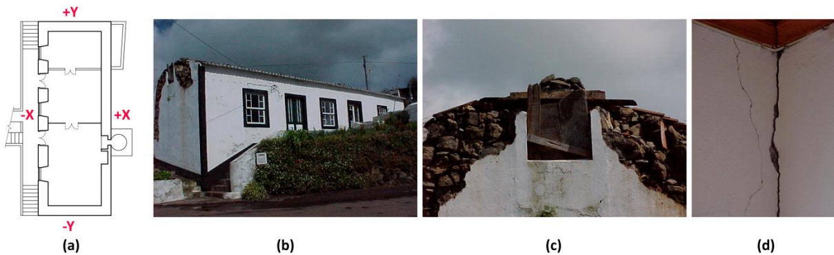
Figure 8.15: (a) Building plan and directions nomenclature; (b) main façade of the building; (c) collapsed gable wall; and (d) visible damage at the wall-to-wall connections from the interior of the building
