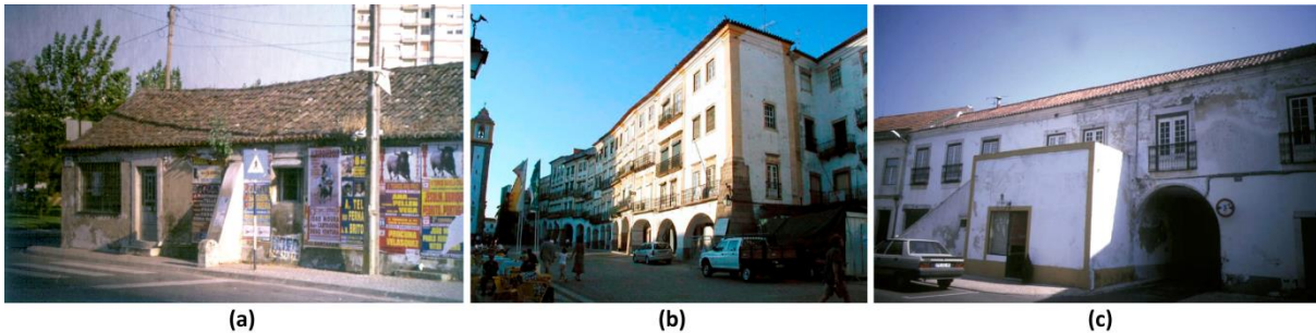
Figure 2.22: (a) Buttress invading the side walk in Samora Correia (Correia and Merten 2001); (b) two-floor buttress in Évora (Correia and Merten 2001); and (c) external staircase in Benavente (Correia and Merten 2001)
