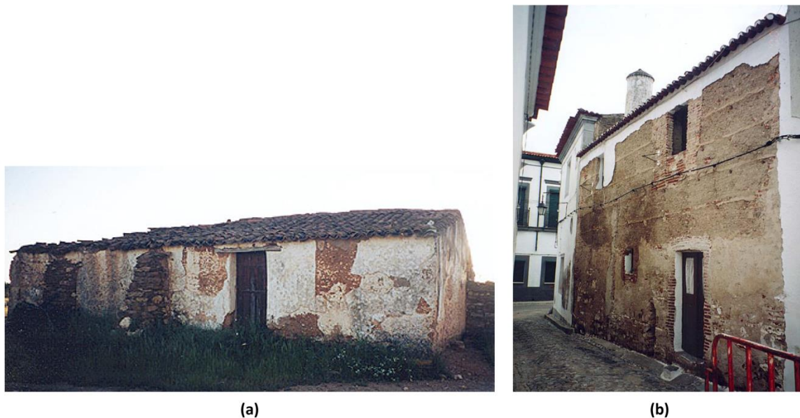
Figure 3.4: (a) traditional rural one-floor rammed earth vernacular construction in Alentejo, Portugal (Correia 2007); and (b) traditional urban two-floor rammed earth construction in Alentejo, Portugal (Correia 2002)
