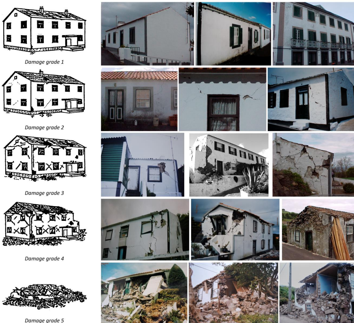
Figure 8.3: Examples of evaluated buildings belonging to each damage grade from the EMS-98 scale
