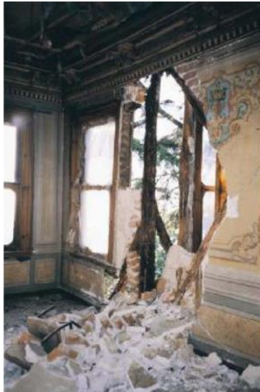
FIGURE 16. DETAIL OF INFILL LOSS AFTER AN EARTHQUAKE [25]
