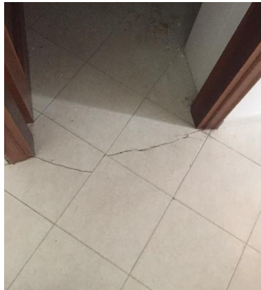
Figure 4.1 Horizontal crack in the WC floor witnessing the autonomous response of the services block
