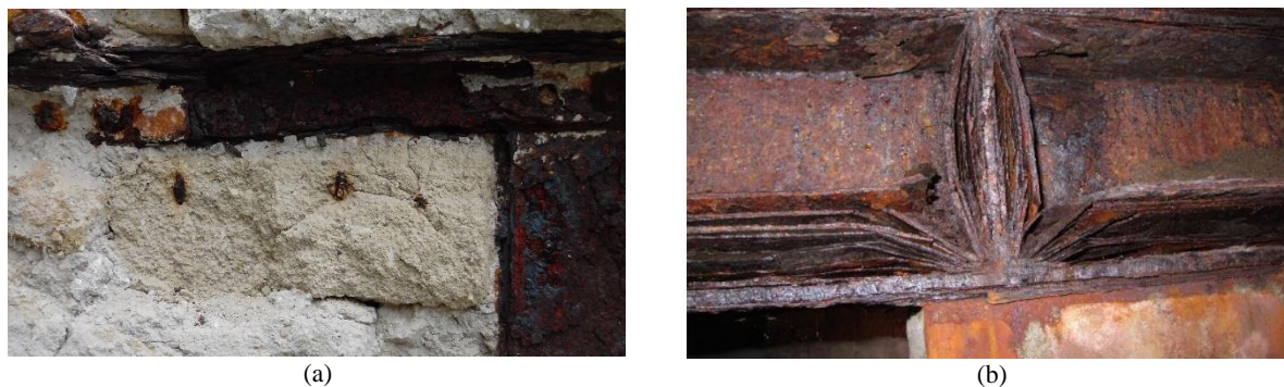
Figure 3.16 Layered corrosion of an horizontal iron element (a), typical delaminated corrosion of a wrought iron element
