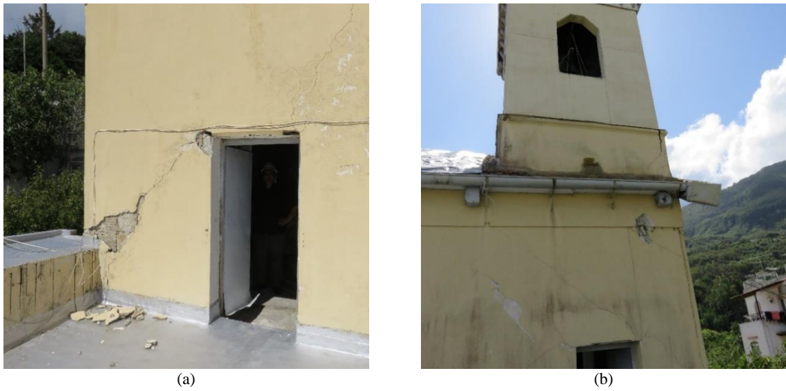
Figure 3.49 Details of the diagonal cracks developed in the South façade at position 1 (a) and in the North façade at position 4 (b)
