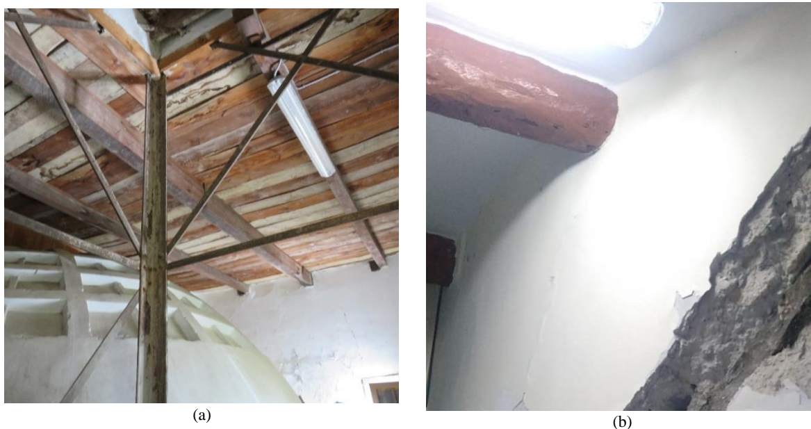
Figure 3.35 Timber floors observed in the resulting space behind the apse at the roof level (a) and at the ground level (b)
