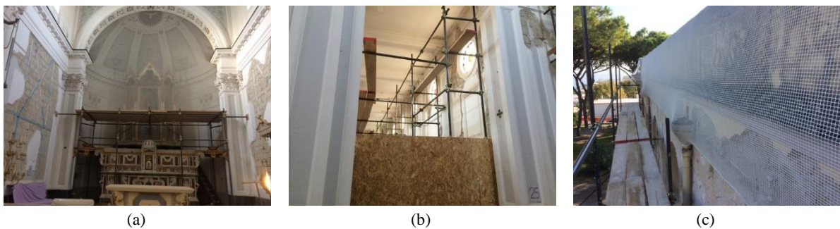
Figure 2.7 Provisional interventions, installation of tube and coupler scaffolding in the apse (a) and in the aisles (b), and application of safety-nets (c)
