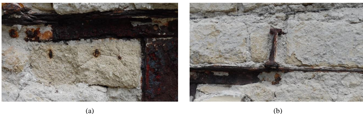
Figure 3.44 Corroded iron vertical and horizontal elements of an iron frame of the church nave wall (a) and the rusting beam end of a floor beam covering the side aisle (b)
