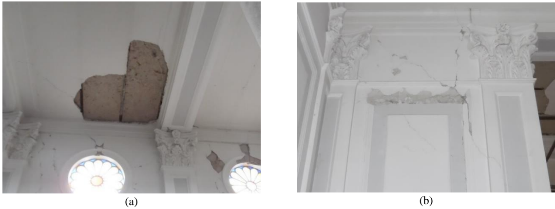
Figure 3.50 Plaster detachment from a ceiling (a) and cracking of a stucco decoration of a capital (b)
