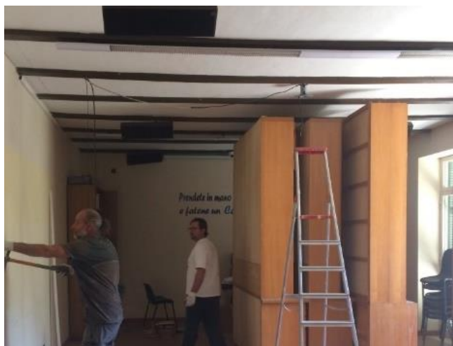
Figure 3.34 Intrados of the iron floor of the parish room in the canonical house
