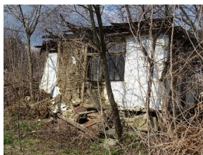
Figure 2.38 Building classified as Type 3, timber-framed with wattle and daub infill in Romania (Dutu et al. 2018b).
