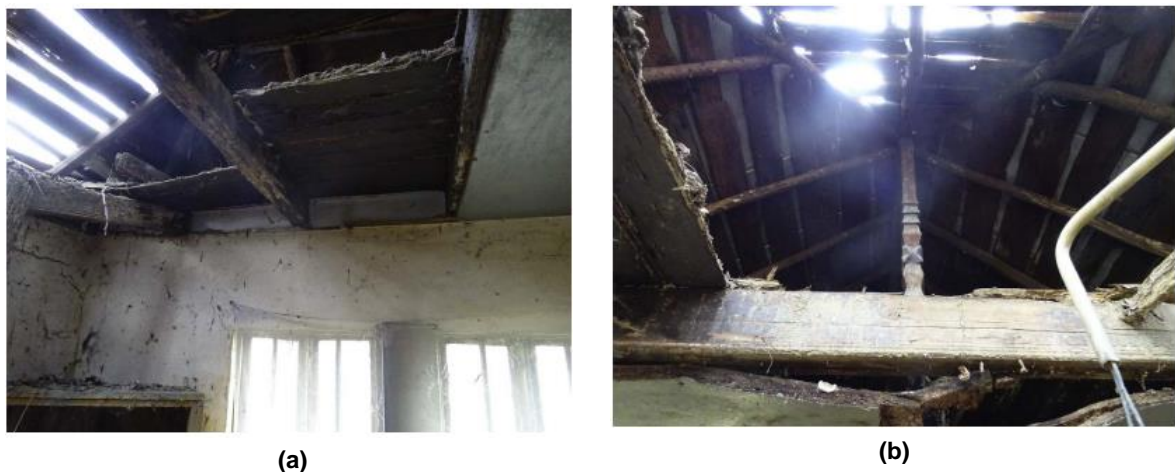
Figure 2.35 Detail of timber floor (a) and roofing system (b) (Dutu et al. 2018b).
