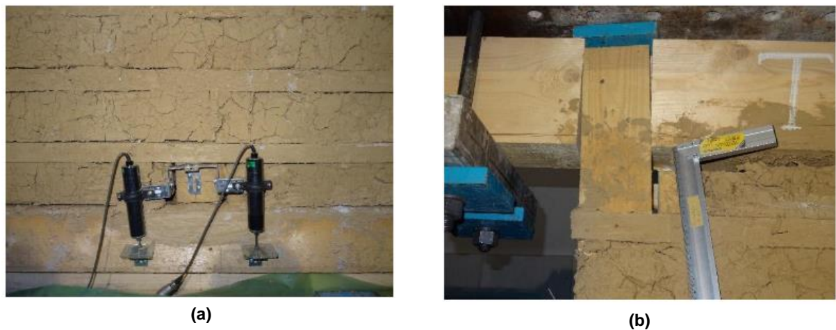
Figure 3.25 S4 damages: central connection with detachment of bracings (a), detachment upper beam (b) (Dutu et al. 2018a).
