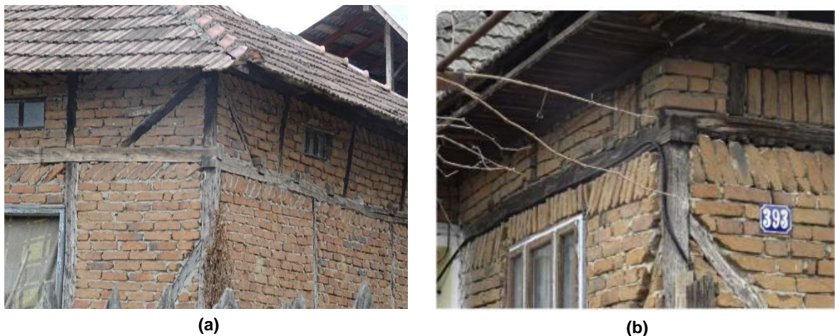
Figure 2.34 Diagonal bricks below the upper beam in Ocnesti (a) and mixed perimeter beam (b) (Dutu et al. 2018b)~.
