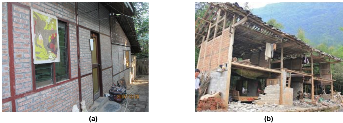
Figure 2.10 House in Myanmar (a) and China (b) after the earthquake in 2016, August 24 th (courtesy of dr. Matsutaro Seki) and the Lushan earthquake in 2013, respectively (Qu et al. 2015).
