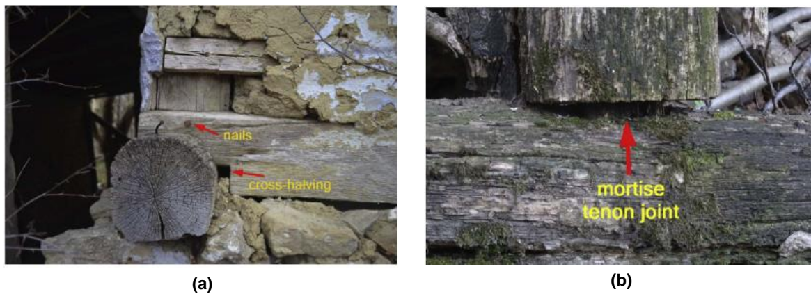
Figure 2.36 Cross-halved (a) and mortise and tenon (b) joints (Dutu et al. 2018b).
