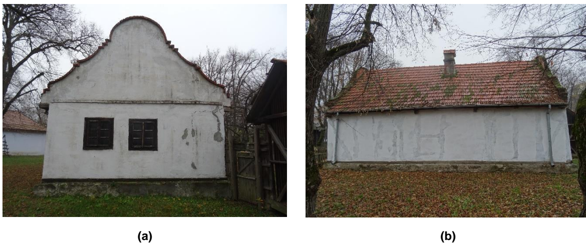
Figure 6.20 Moisture-related problems in TW4 (a) and LW1 (b) walls.
