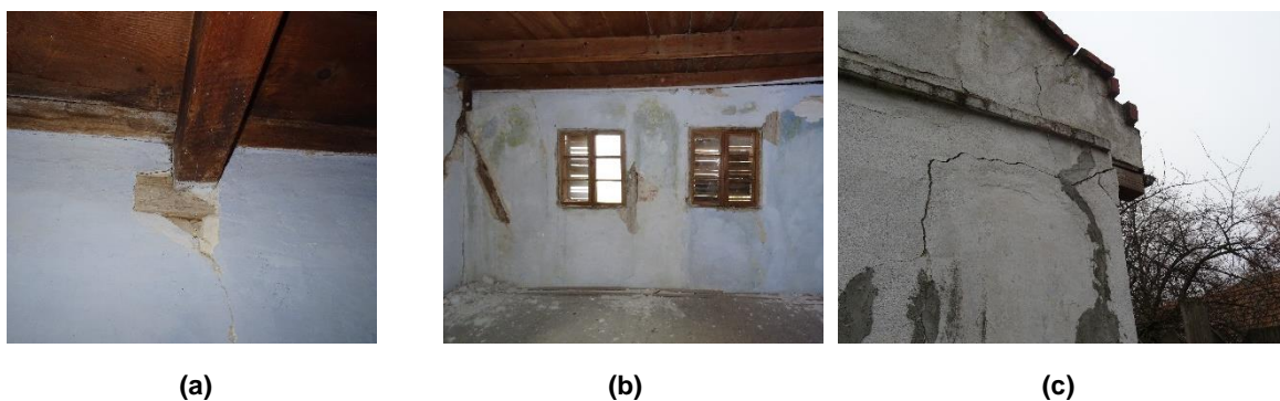
Figure 6.18 Minor cracks (a), detachment of plaster (b) and crack of masonry infill (c).
