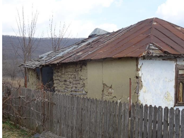
Figure 2.39 Building classified as Type 4, timber-framed with mud mortar infill in Romania (Dutu et al. 2018b)).
