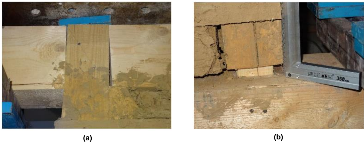
Figure 3.24 S4 damages: compression perpendicular to grain (a), uplift of external connection (b) (Dutu et al. 2018a).
