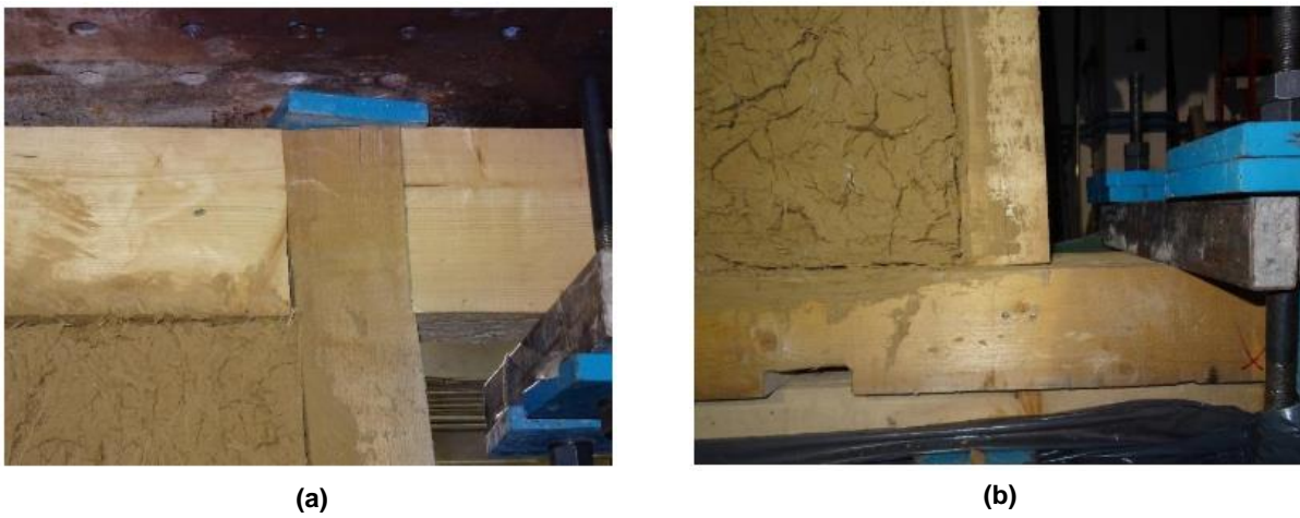
Figure 3.22 S3 damages: compression perpendicular to grain (a), small uplift external connection (b) (Dutu et al. 2018a).
