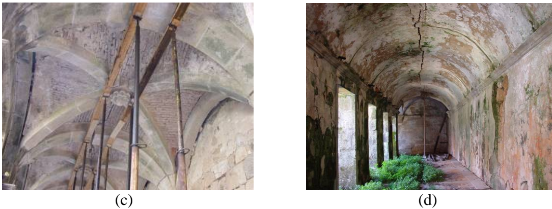
Figure 13 – Damage in the Salzedas’ cloister: (a) mapping of cracks (2 nd level); (b) out-of-plane displacements; (c) aspect of vault (1 st level); (d) aspect of vault (2 nd level).
