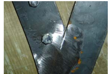
(c) Stirrup failure
