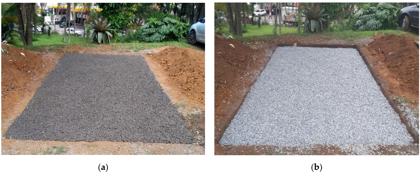
Figure 4. Parking space lined with recycled concrete aggregate (RCA)-based pervious concrete (a) and seated sub-base layer (b).
