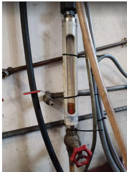
Figure 40 - Water Flow meter.
