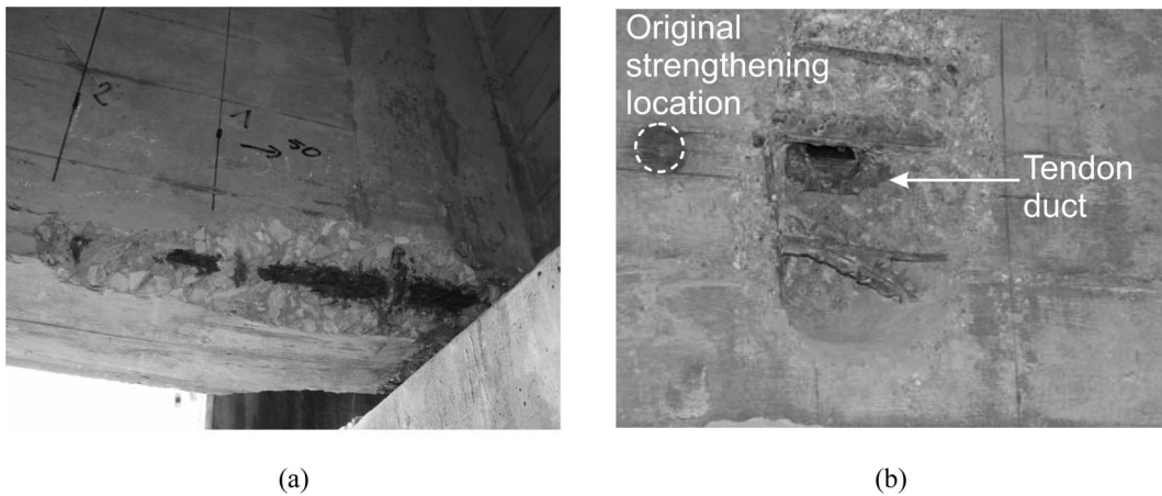
Figure 6. Example of: (a) corrosion of the reinforcement in the Barra Bridge, and (b) window opened in a longitudinal beam for the detection of tendon ducts in the Lanheses Bridge.
