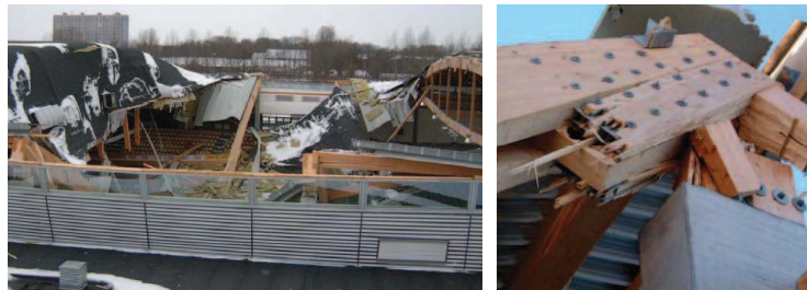
a) An intact truss is seen to the right b) Rupture at the critical cross section in the corner connection
