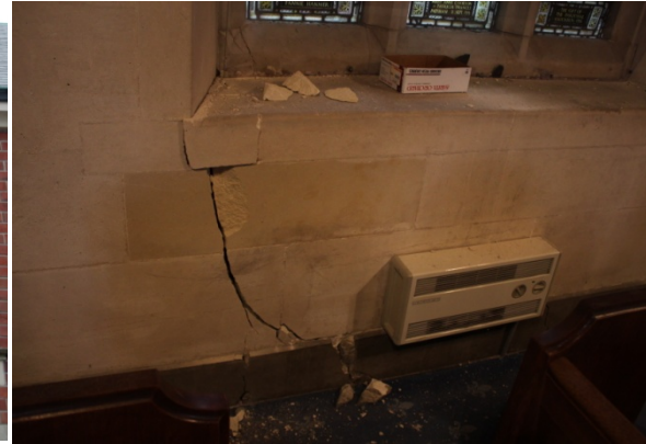
(b) shear damage in the longitudinal walls (mechanism 6), inside (St. Barnaba's, stone, Fendalton)
