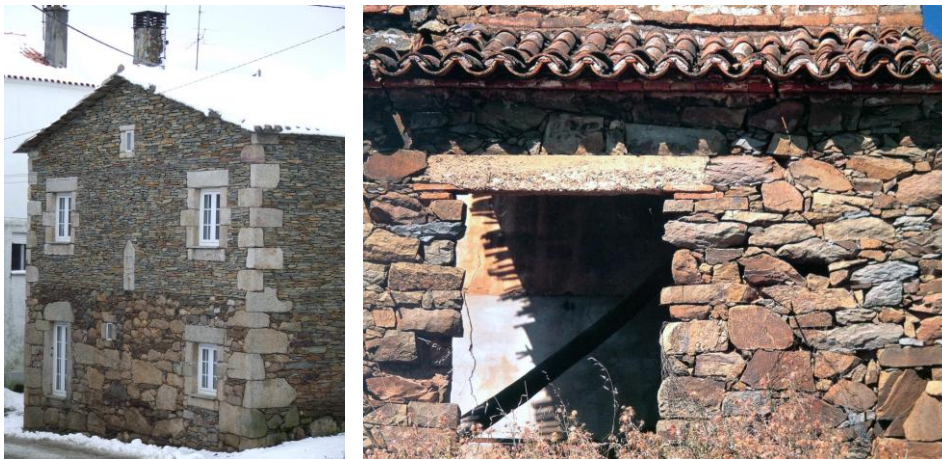
Figure 3. 8- Supporting granite elements in corners of schist constructions, Figure 3. 9- Supporting granite elements over openings. (From: Casella, 2003)
