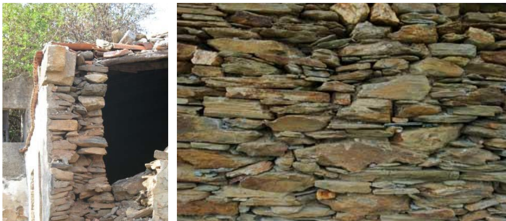
Figure 3. 6- Section of a double leaf schist masonry wall with connectors, Figure 3. 7- Elevation of a schist masonry wall (From: Oliveira, 2003)
