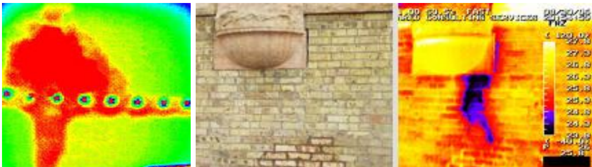
Figure 2. 6- Detection of interior metal bars via infrared thermography, Figure 2. 7-Inspected wall geometry, Figure 2. 8- Moisture detection of the inspected wall via infrared thermography
