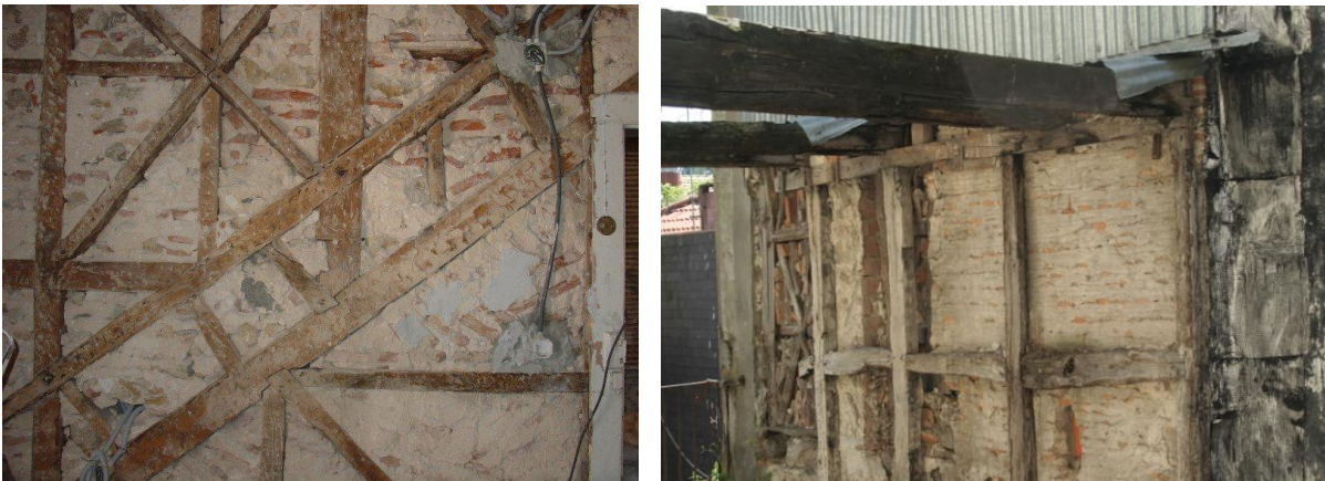
Figure 3. 15- Brick masonry between timber elements in Gaioleiro walls, Figure 3. 16- 'Tabique' exterior walls with no diagonal timber frame, (From: forumdacasa.com , sjoaohostel.wordpress.com )
