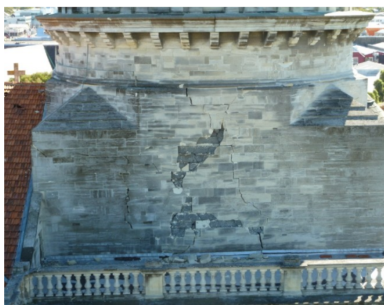
Figure 33 – Damage to the South supporting wall of rotunda.
