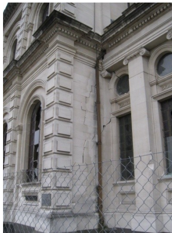
Figure 28 – Shear cracks in the transept-main nave connection.
