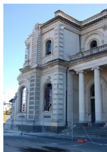
Figure 24 – Detail of the West wall collapse of the South bell tower.
