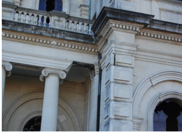
Figure 26 – Detail of shear cracking around South transept window and local collapse of the architrave.
