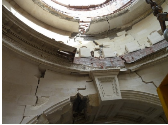
Figure 39 – South arch severe damage.
