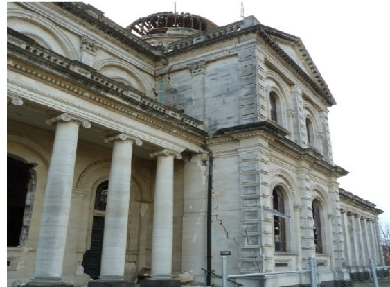
Figure 41 – Developing of a diagonal block failure in the South transept façade.
