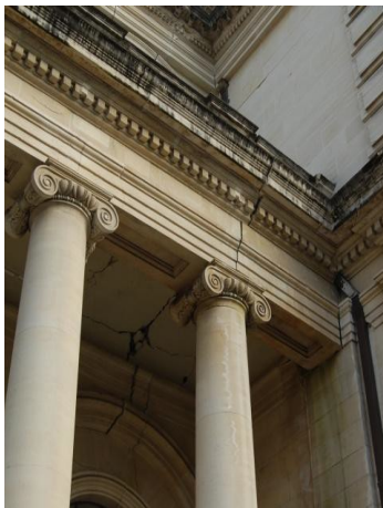
Figure 27 – Large diagonal crack in the entablature near to the north transept.
