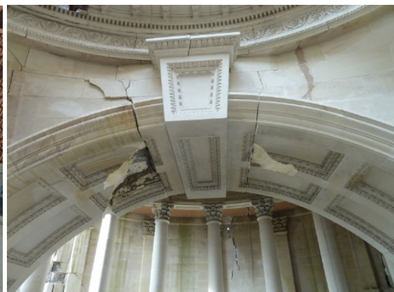
Figure 37 – Damages to the key stone of the East arch.
