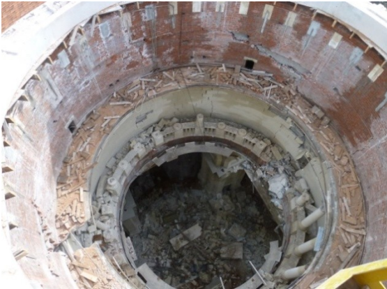
Figure 40 – Visible damage to the main dome drum (after the removal of the internal dome in 25 August, 2011).
