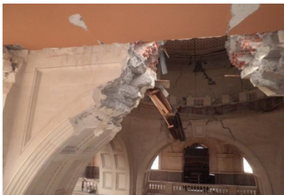
Figure 30 – Collapse occurred in the north arch of the sanctuary.
