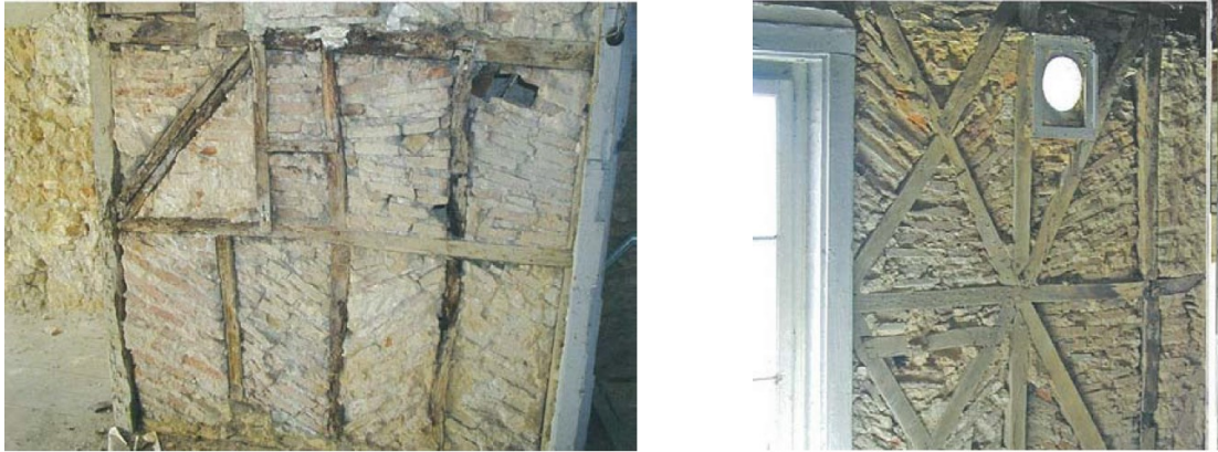
a) b) Figure 8 – Wall system in Lisbon: (a) Before the earthquake; (b) After the earthquake, where an x-braced internal wooden frame is clear.
