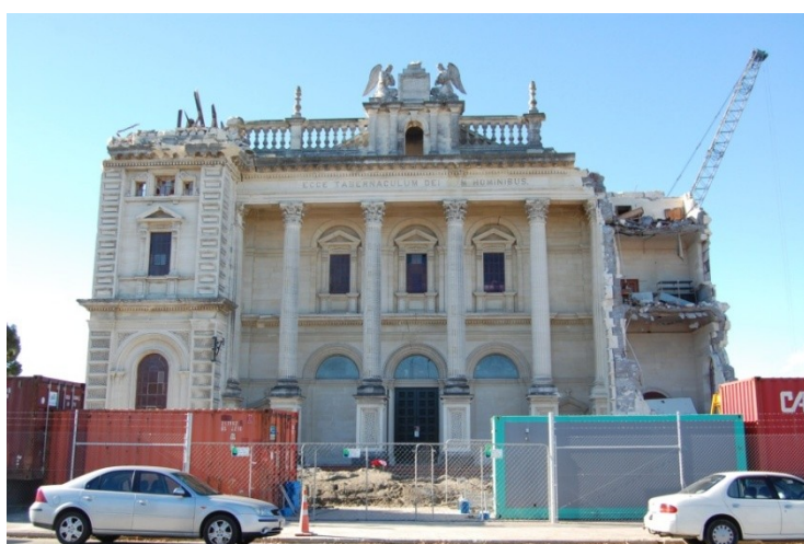
Figure 23 – West façade of the Christchurch Catholic Basilica and the damage in the two bell towers, North (left) and South (right).
