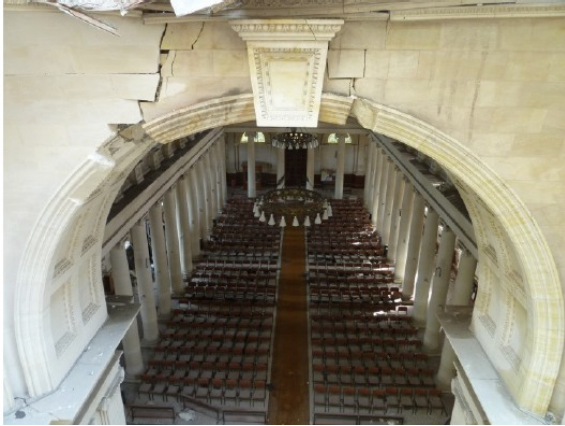
Figure 38 – Damage along the West arch.
