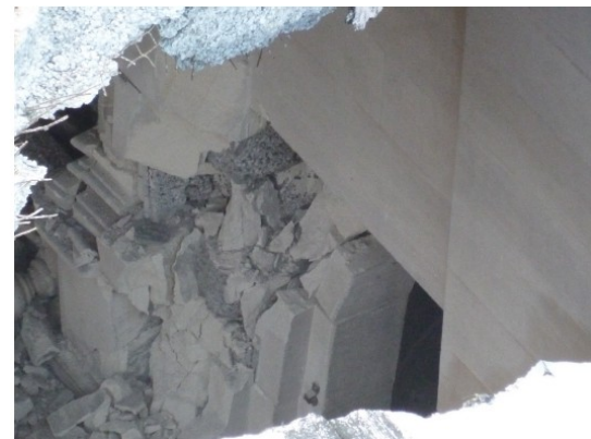
Figure 42 – Crushing of the top South-West column.
