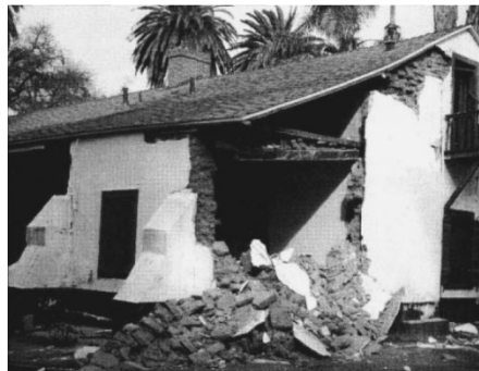
Figure 4: Partial collapse of a house at Rancho Camulos in California, USA, after the 1994 Northridge earthquake /13/.
