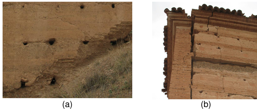
Figure 2. Structural damage in earth constructions [15]: (a) basal erosion; (b) cracking.
