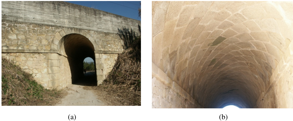
57 Fig. 1. Typical skew masonry arch constructed using the English method: (a) front view; (b) detail 58 of the intrados
