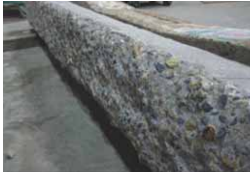
Figure 5: Abrasion of 30 years old heavy haul sleepers
