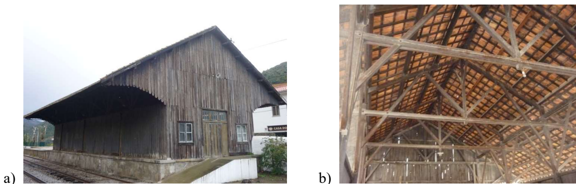
Figure 1: Timber warehouse: a) main façade and lateral façade oriented to the railways; b) view of the roof by the interior.
