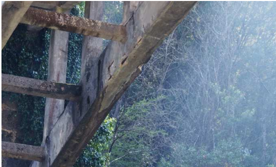
Figure 2. Detail of one of the damaged arch girders
