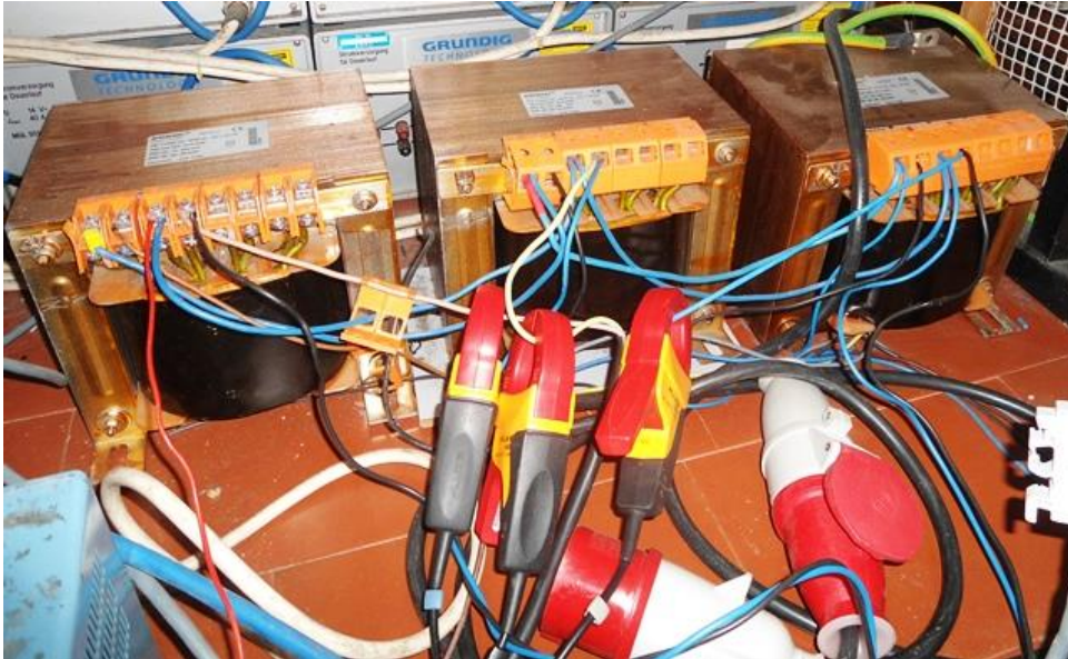
Figure 5.22 – Transformers used to reduce the levels of the voltages supplied by the electrical grid.
