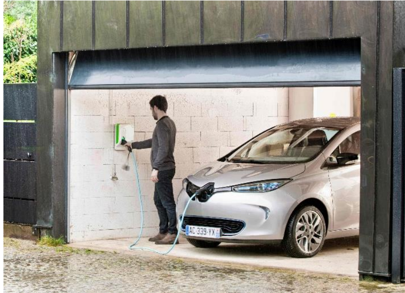
Figure 1.11 – Charging of a Renault ZOE , using a dedicated EV supply equipment installed (gently provided by Renault Portugal ).
