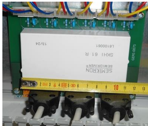
Figure 5.19 – PCB developed in the GEPE for the driver circuit of the IGBTs.
