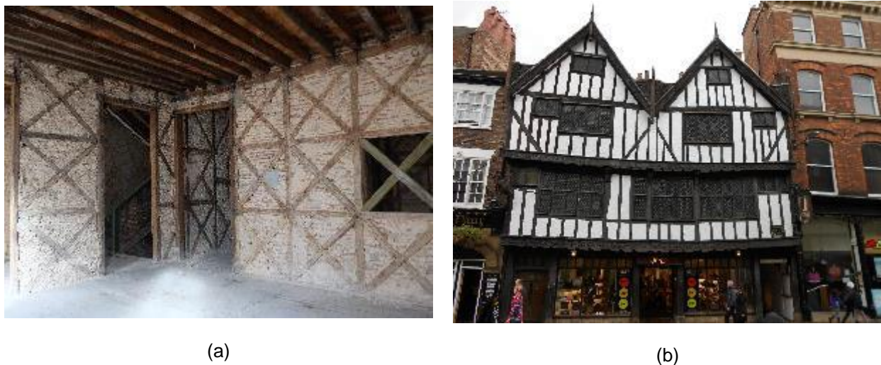
Figure 1 (a) Frontal walls in (a) Pombalino building (© Stellacci) and (b) timber-framed house in York, UK, XVI century (© Poletti).
