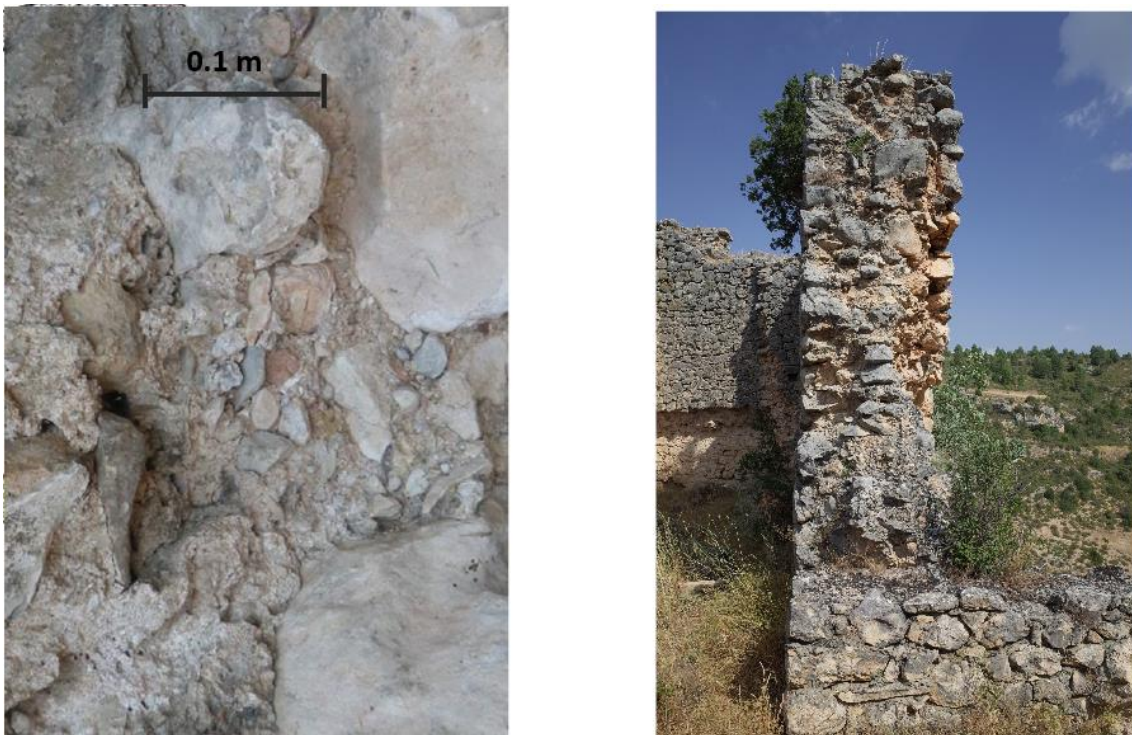
Figure 19: Broken wall exposing inner leaf and Inner leaf of the masonry wall
